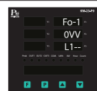
Display Previous Fault Output 1
