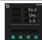
Display Previous Fault Output 2
